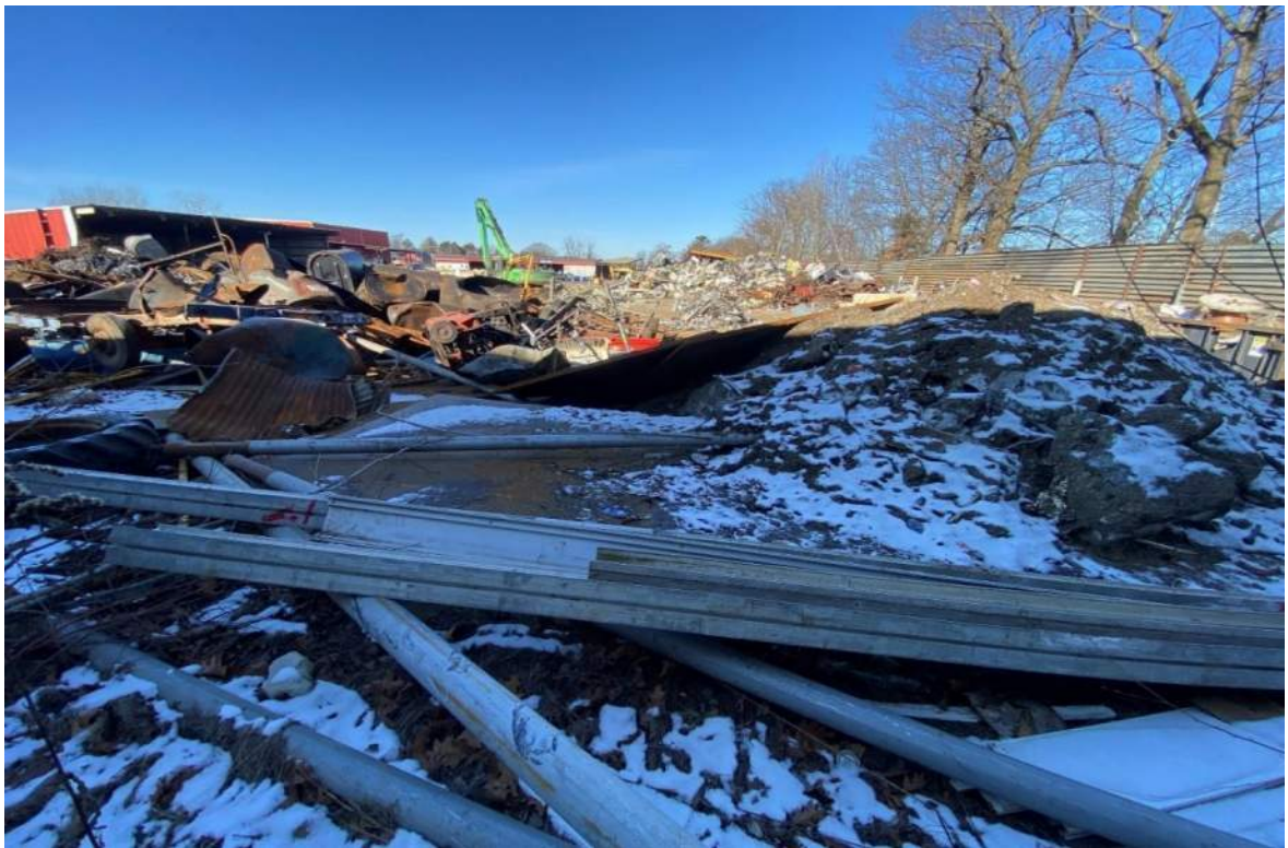
Photo 7: Refuse pile, facing East.
